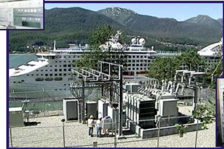
Alaska Electric Light & Power shore side power station, Juneau, Alaska
