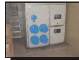
Vessel Power Management System with Patton and Cooke C150 Receptacles
